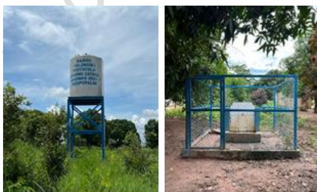
Figure38 - Community water supply system in Pelengue 2
